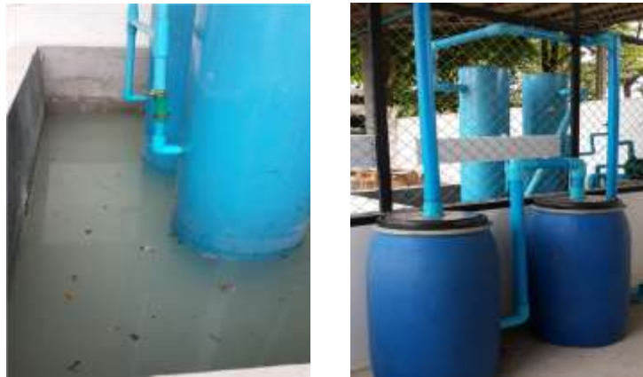
Fig. 4: Biogas Purification with Limestone Solution (left) and Steel Wool (right) before Going into the Generator.
