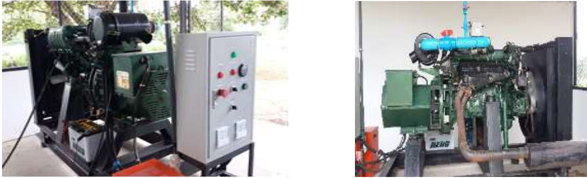
Fig. 5: A Modified Generator for Three-Phase AC Electricity Using Biogas Fuel.
