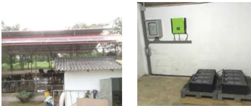
Fig. 6: Rooftop Solar Photovoltaic Panels on the Dairy Barn (left) and the Hybrid Inverter Connecting to the Grid and Batteries.
