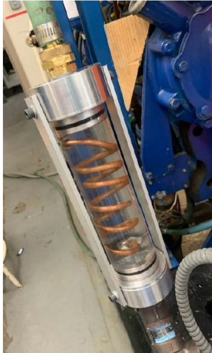
Fig. 6. testing one of the heat exchangers on the diesel engine
