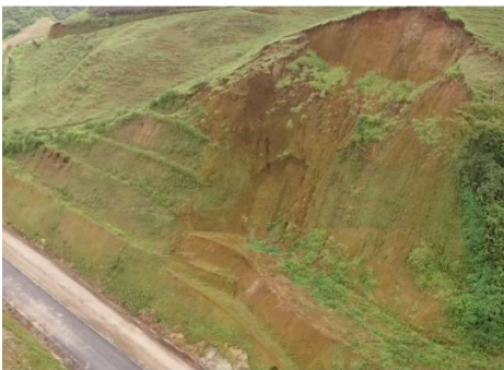
A. Intervention and failure, slope at km 17.
