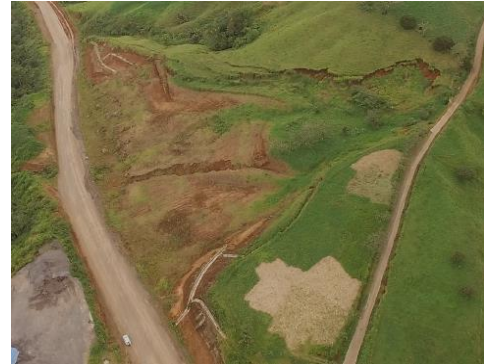
B. Slope on km 29
