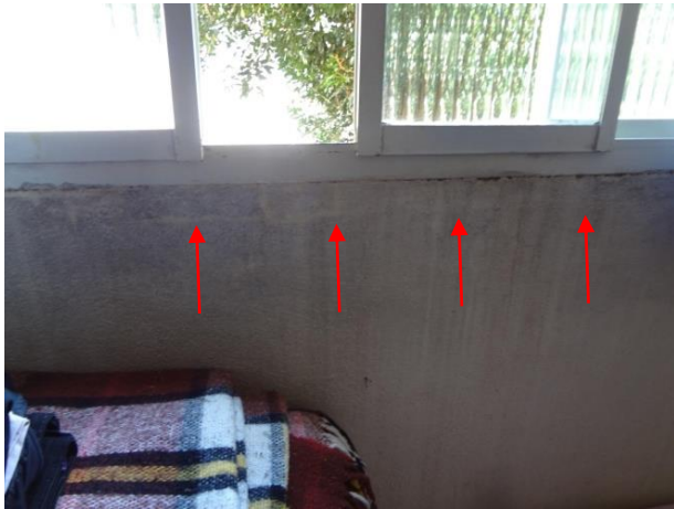
Fig. 4: Recurrent infiltration through the HIS window.
