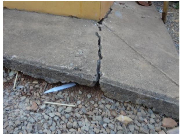
Fig. 5: Cracks in the HIS ride.
