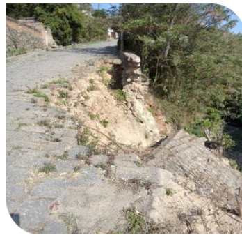
Figure 5: Signs of instability (triggering landslide).
