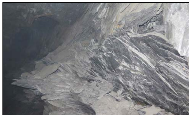
Fig. 4: Creep buckling of the pelites at some galleries in Draa Sfar mine
