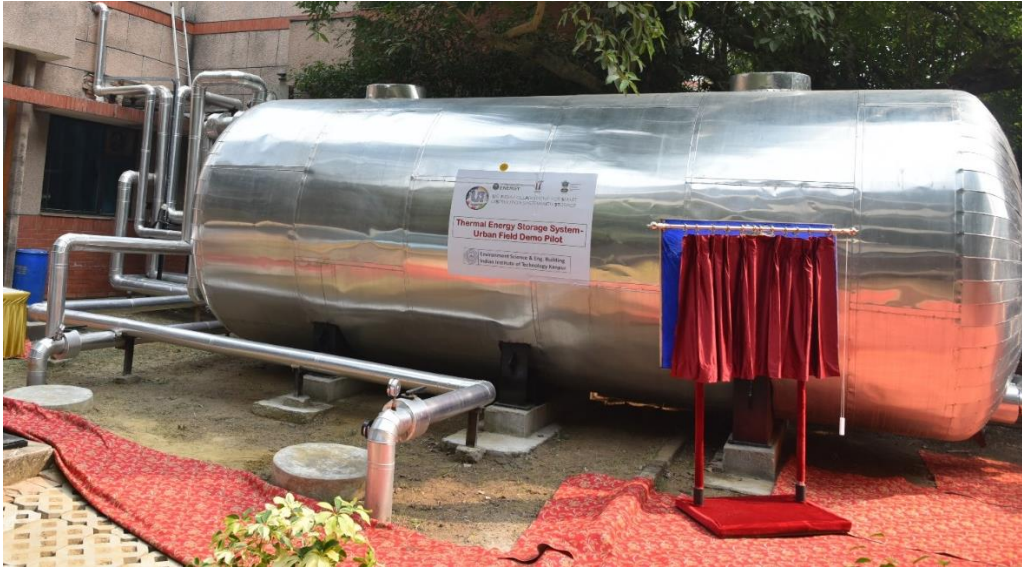
Fig. 3: Thermal Energy Storage System Horizontal Outside Tank
