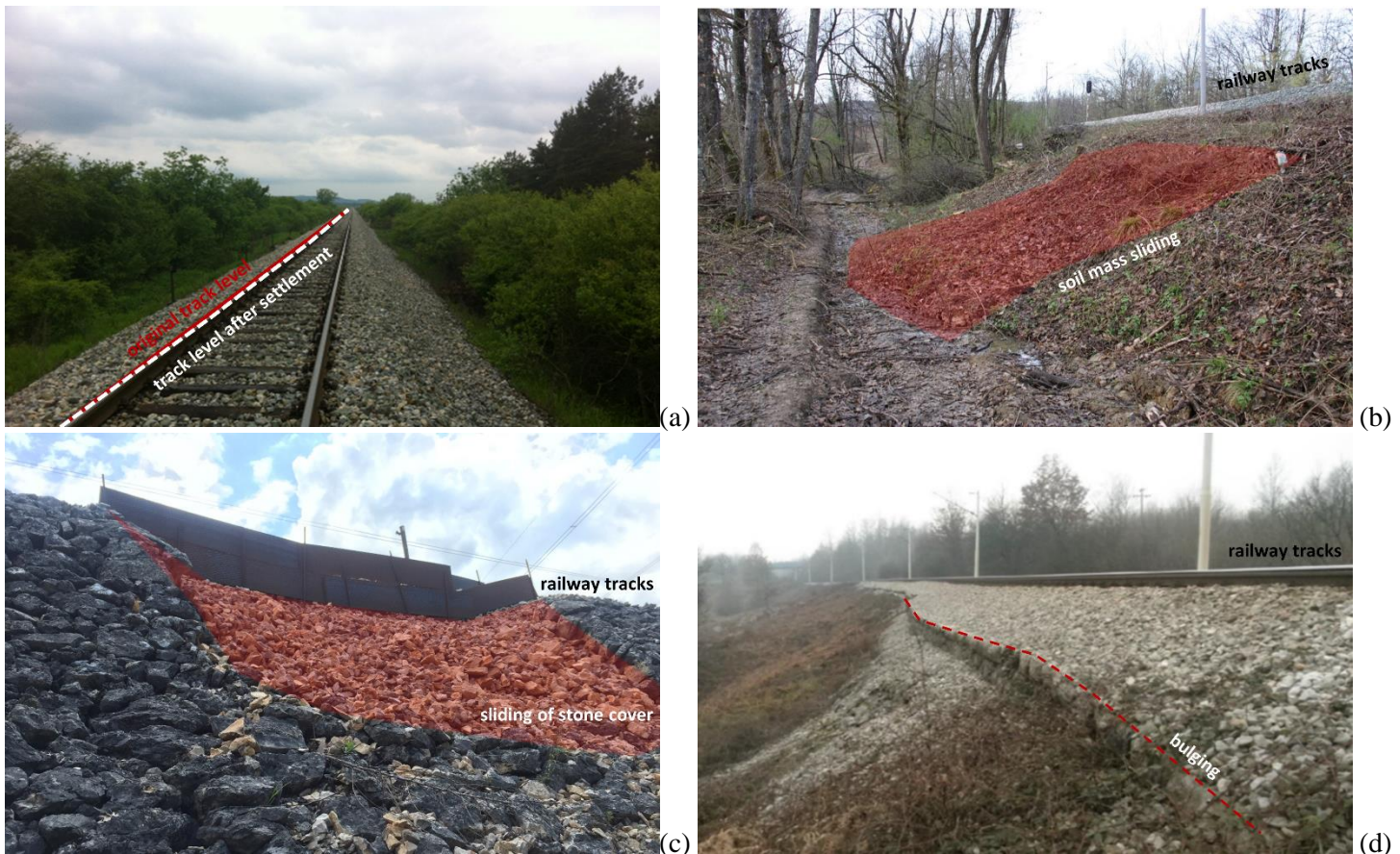
Fig. 2: Some of embankment-related issues: (a) large settlements, (b) overall stability loss, (c) sliding of slope stone cover, (d) settlement and stability issues due to poor drainage
