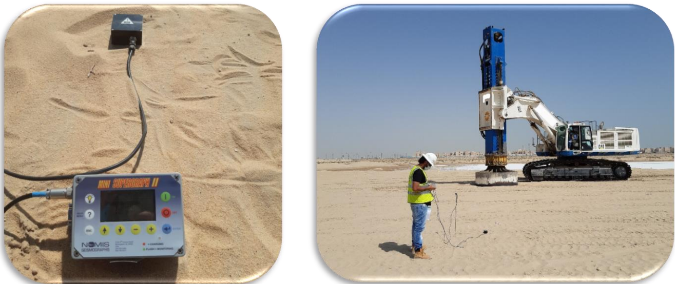
Fig. 2: Vibration Recording Device and Field Photo
