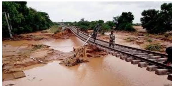
Fig. 1: Washed out embankment under railway tracks during 2017 floods.
