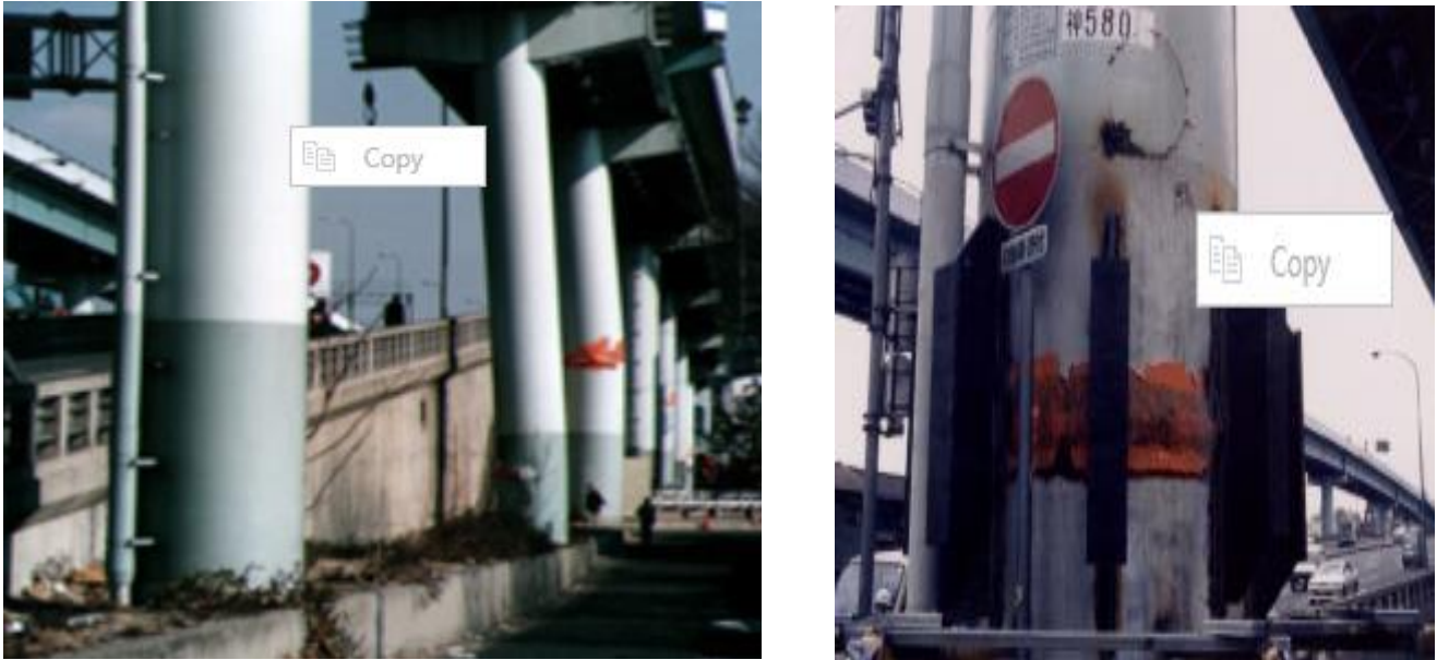
Fig. 1: Local buckling of steel bridge pier, Kobe Earthquake, January 1995.
