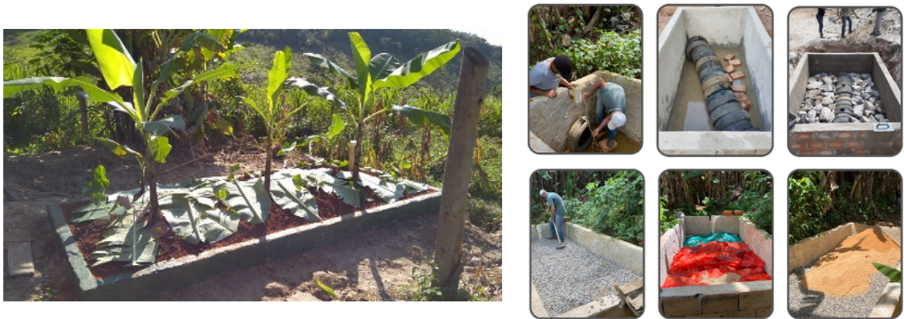
Fig. 3: Evapotranspiration System (TEvap) using concrete chambers filled with stones, tires, sand and soil that receive the sanitary sewage. Banana plants ( Musa sp ) are responsible for nutrient absorption and water transpiration.
