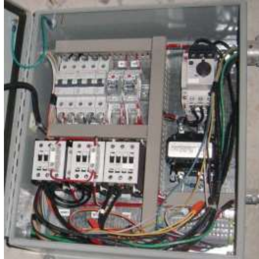
Fig. 7: Test rig system control box.
