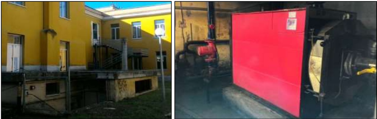
Fig. 4: Centralized Heating Plant a) External view; b) The boiler.
