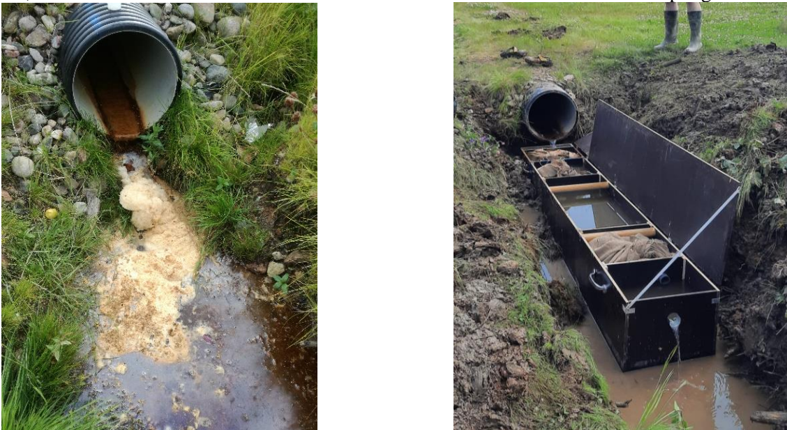
Figure 3: Contaminated run-off water outlet (left) and installation of a passive barrier filtration system (right).
